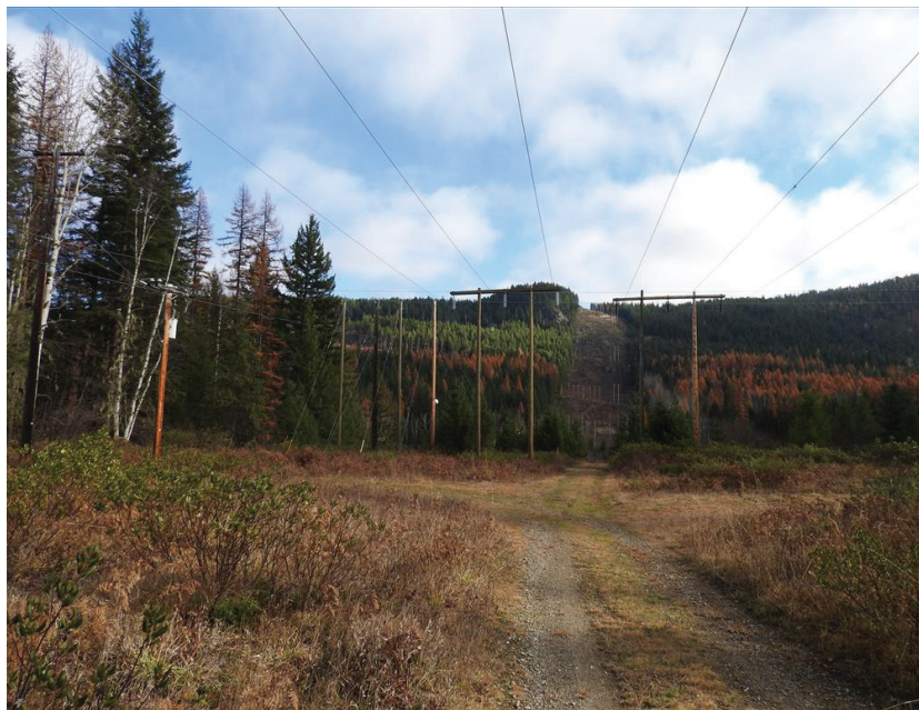
Distribution crossing on the 6OL210 Transmission Line.
