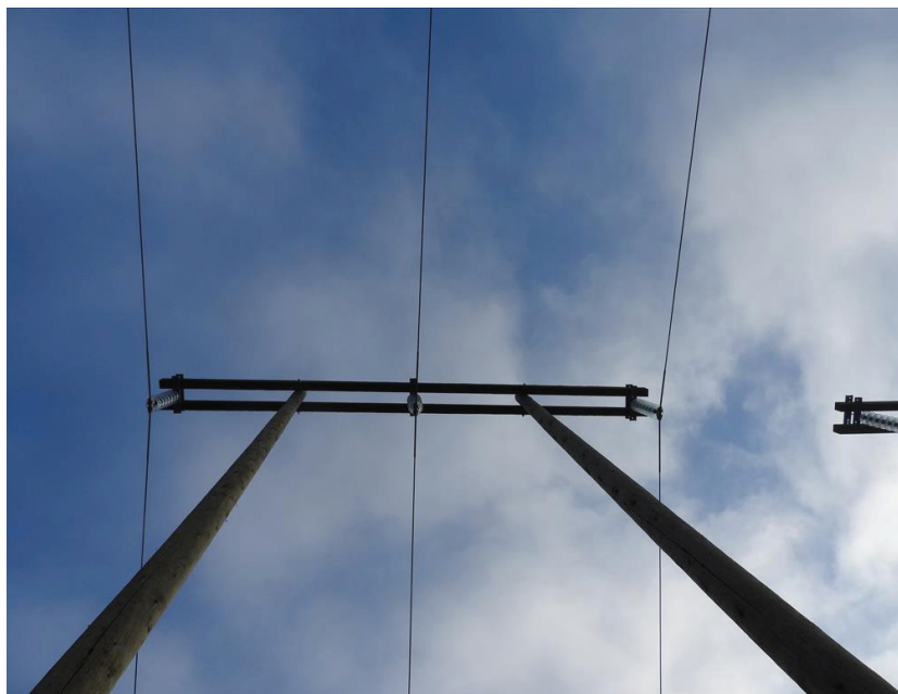
6OL210 Transmission Line.
