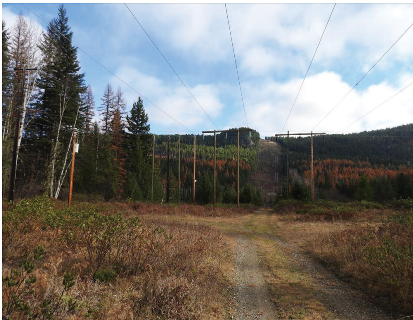
Distribution crossing on the 6OL210 Transmission Line.
