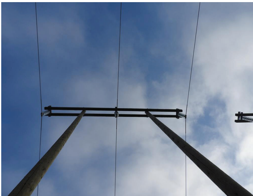
6OL210 Transmission Line.
